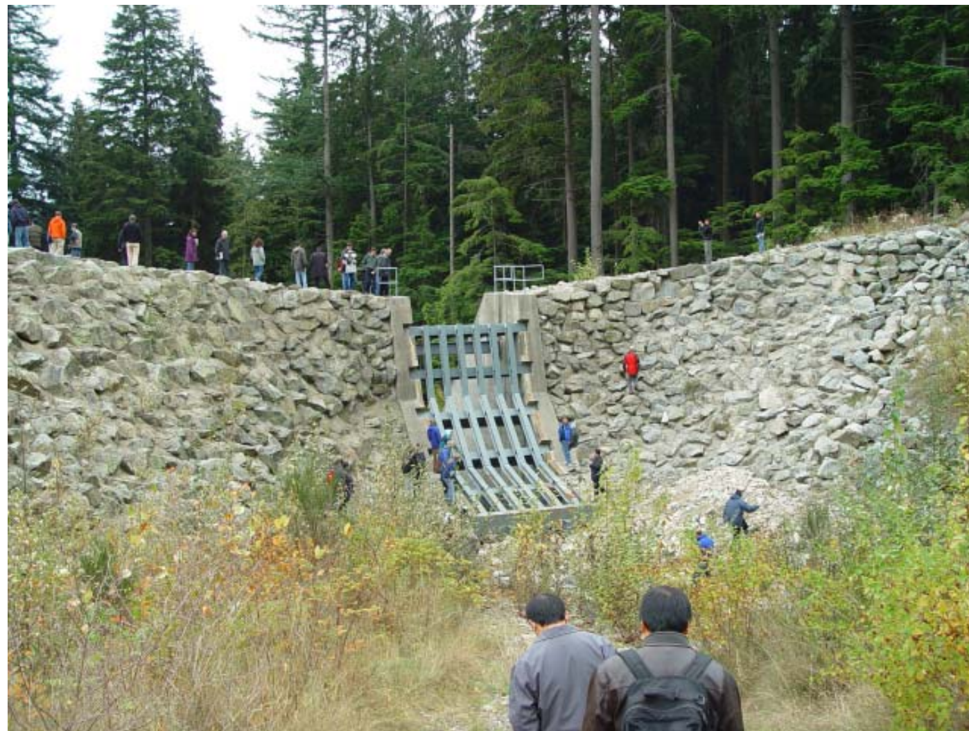
A debris-detention basin outflow structure protecting a suburb of Vancouver, Canada. A similar structure may be feasible in the old quarry just up the Awatarariki Stream.
